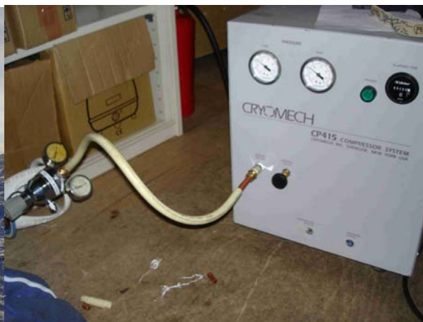
He bottle connected to the He compressor via the pressure reducer when attempting to refill the He tank
